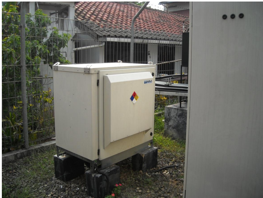
Figure 10: Fuel cell system deployed by Idatech on Java
