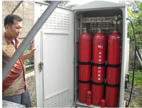
Figure 4.1: Hydrogen storage cabinet at telecoms site in Indonesia. Each bottle contains enough hydrogen to generate 7kWhr electricity.
