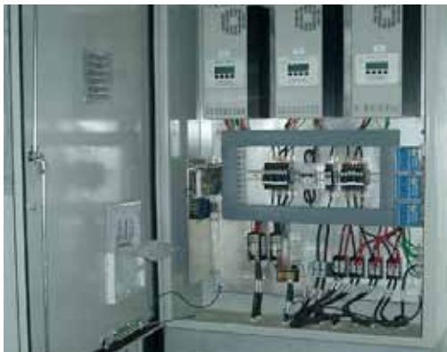
Apollo Solar PV for Telecom System® in IP66 Enclosure
