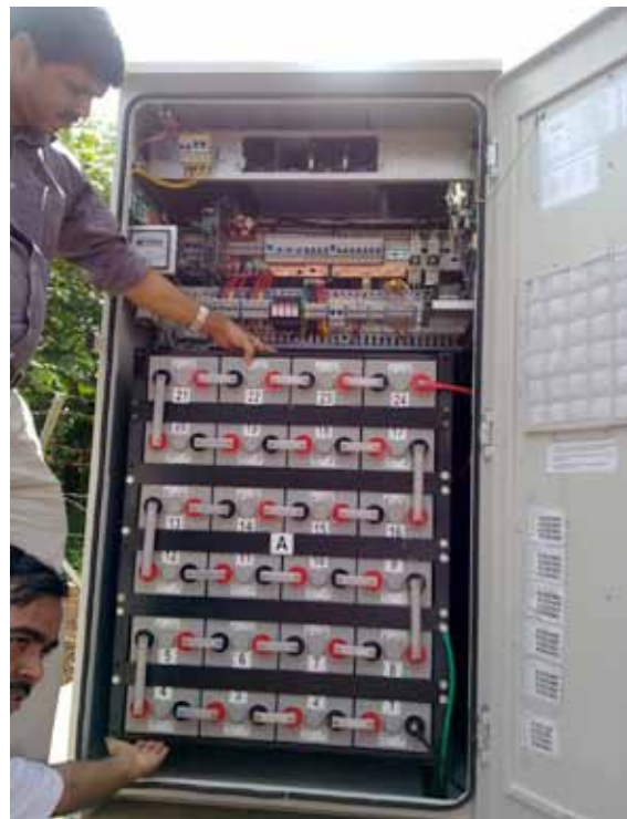
Figure 1: Alternating Mode: Smart Energy Controller & Cycling Batteries at VF-Essar Sites in India
