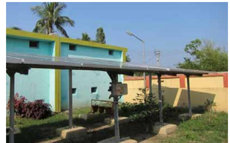
Bushlight India's solar array and power house
