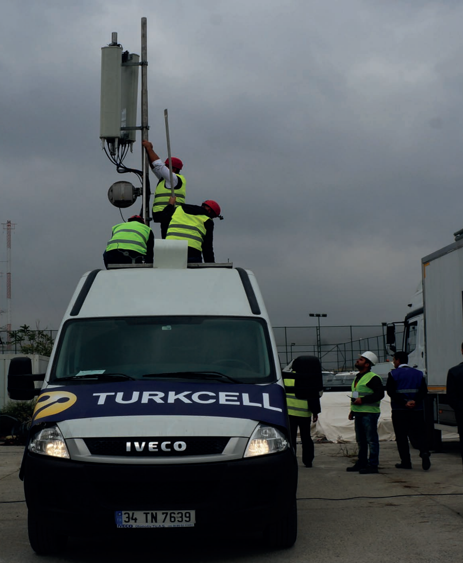
Turkcell at the Istanbul earthquake simulation – a Mobile BTS undergoing set-up
