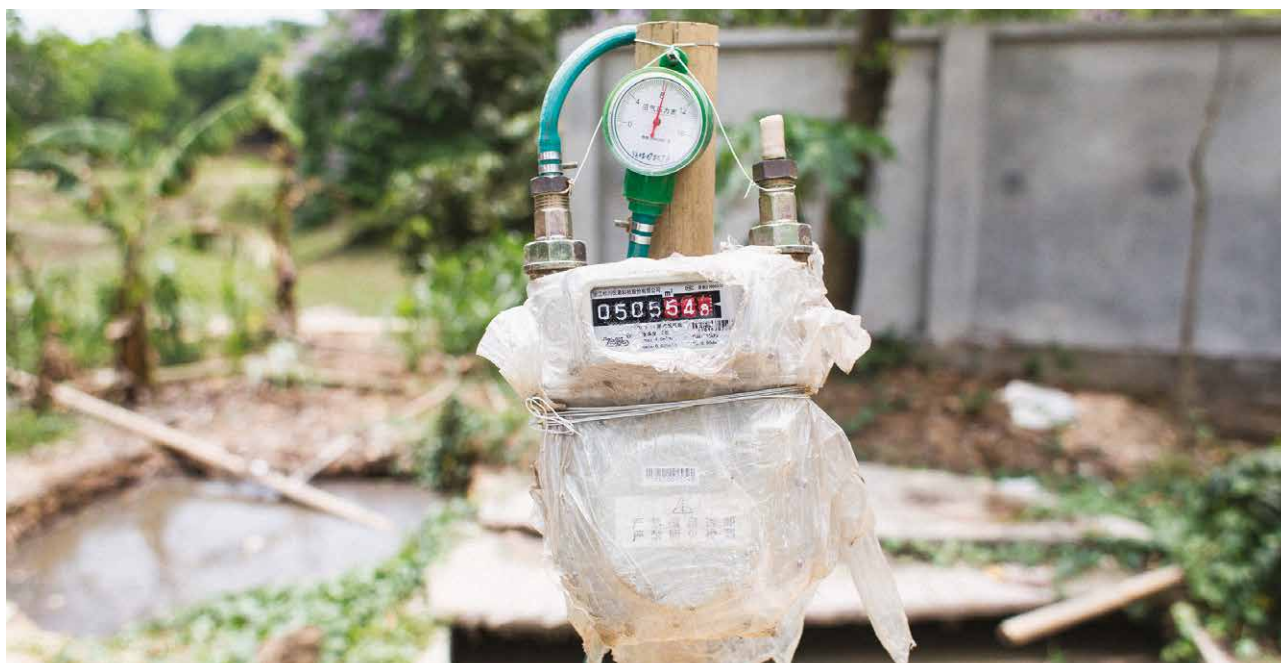
Gas meter at Site 1 indicating normal pressure in the digester
