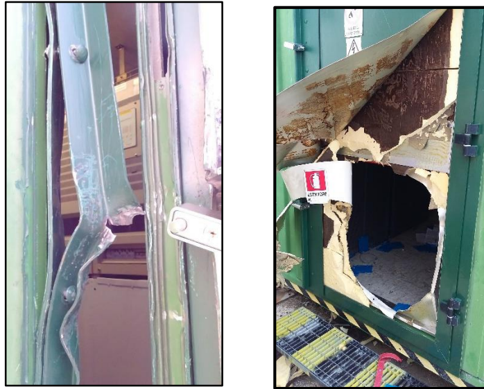
Figure 4: Battery Shelter at Mast sites: Entry broken to entry and forcibly remove batteries.
