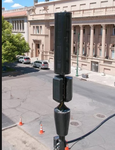
3 sector street site with lower band canister antenna
