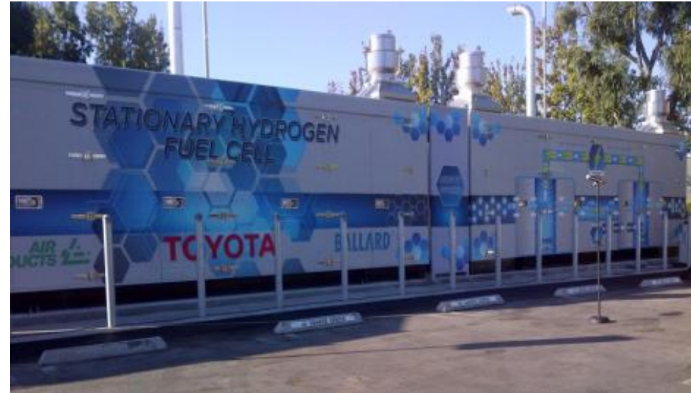
1MW ClearGen™ system at Toyota campus – Torrance, CA
