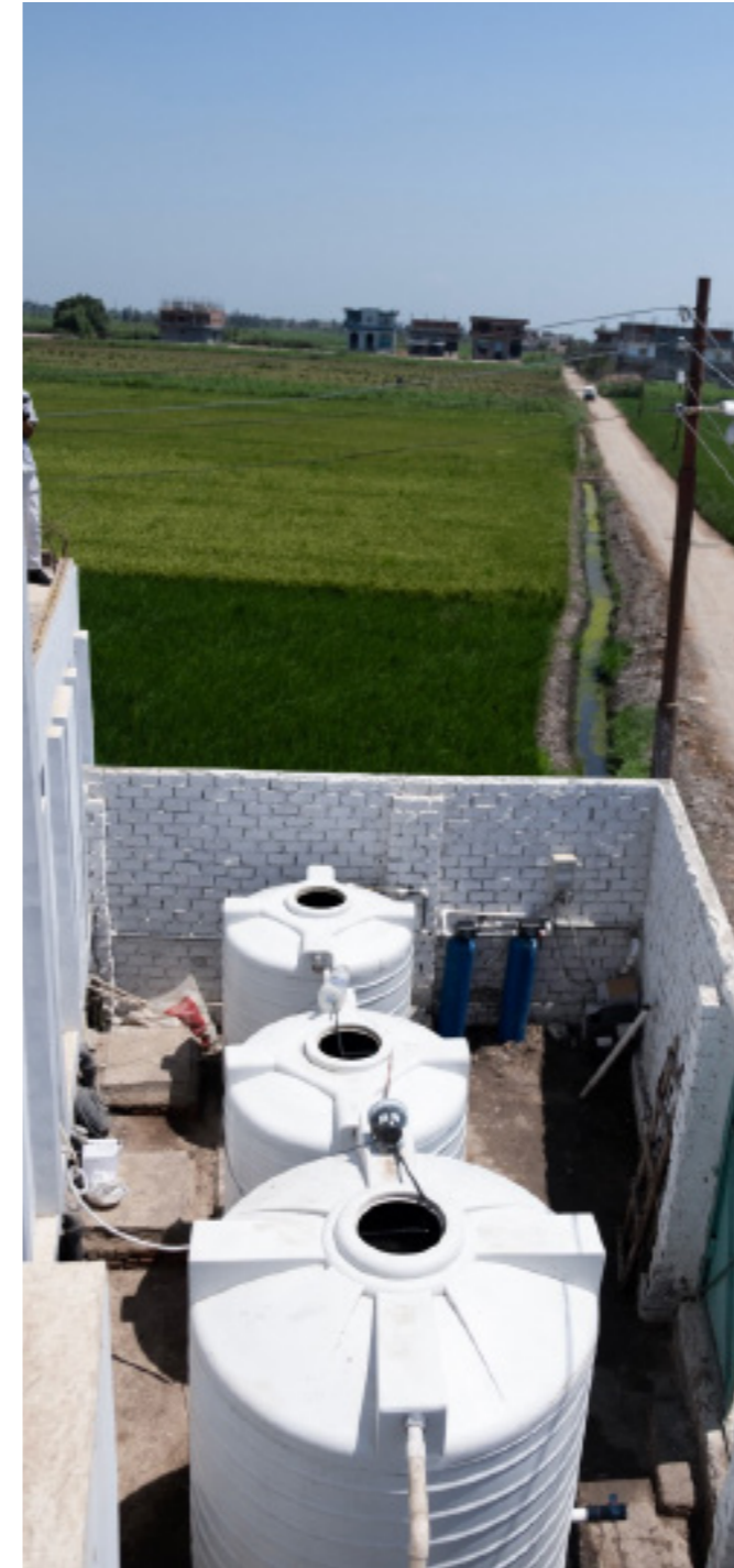
Figure 2 SuWaCo's modular plug-and-play wastewater treatment technology deployed on site
