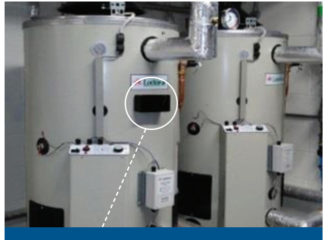
Figure 10: A connected monitor from Horus attached to factory equipment
