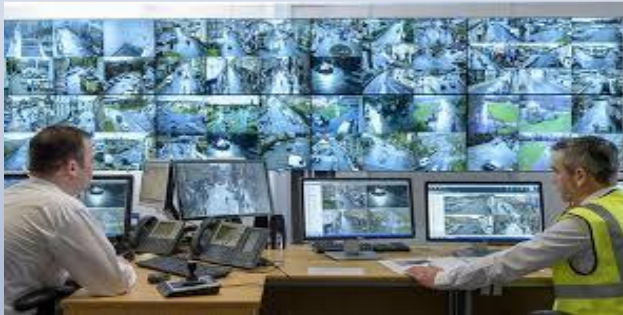
Traditional CCTV control room (reactive)
